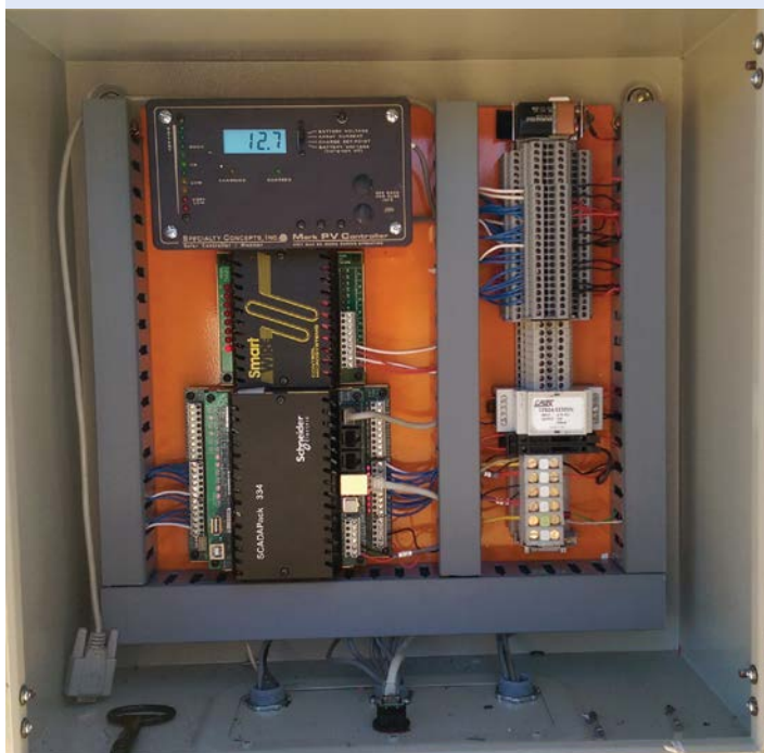
Garden Control System
